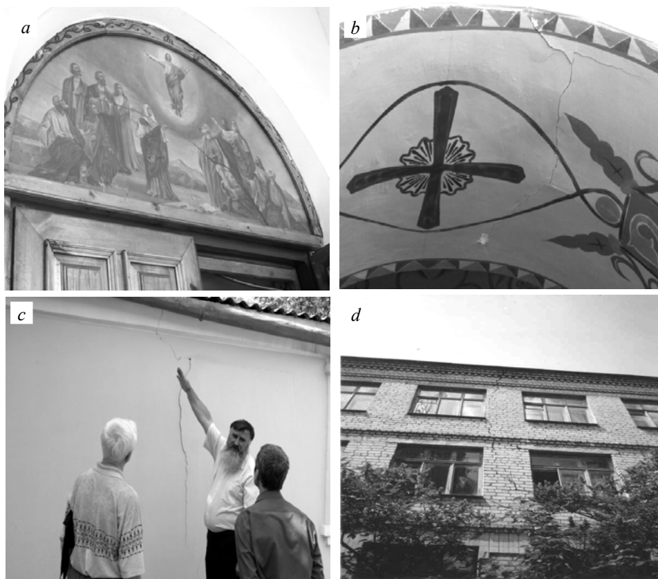
Fig. 2. Instances of buildings damages due to industrial explosions in Kryvyi Rih (photographs by Iurii Kaliukh)
